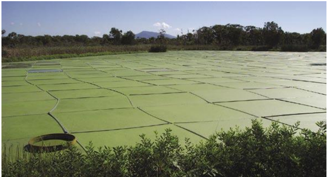
Figure 12: Harrington sewage treatment plant, duckweed and grid (1)
